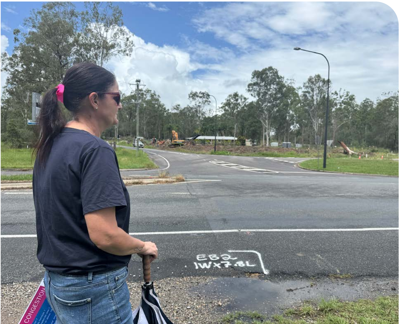
Cr Natalie Willcocks on the site of the major intersection upgrade at the entry into Flagstone.
